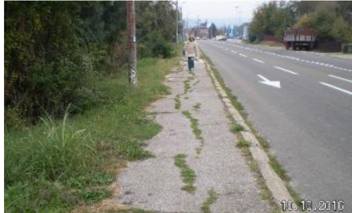
Picture 14. Detail of the sidewalks in the zone of the state road IB 25
