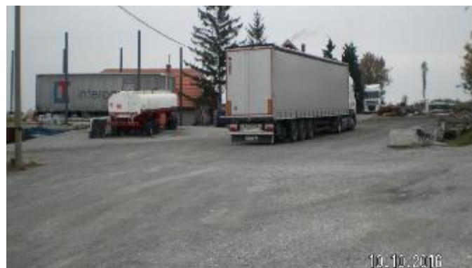
Picture 28. Work zone on the left side of the road, next to landslides
