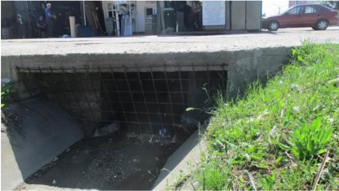
Figure 5. Negotin – transition in piped part of the canal (The location where open canal transits in piped canal)
