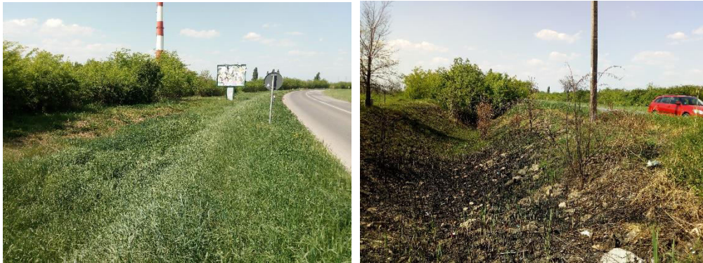
Figure 4. Intake canals on the right side of the road on the subject road section
