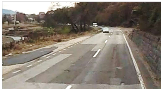
Picture 45. Damage of pavement
