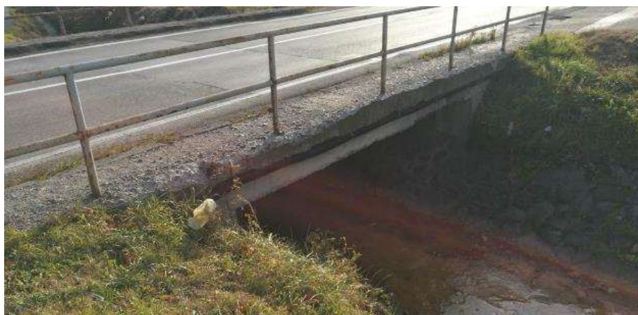
Pictures 11 and 12: Bridge over the stream near the Ibar mine (stat. km 221 + 416)
