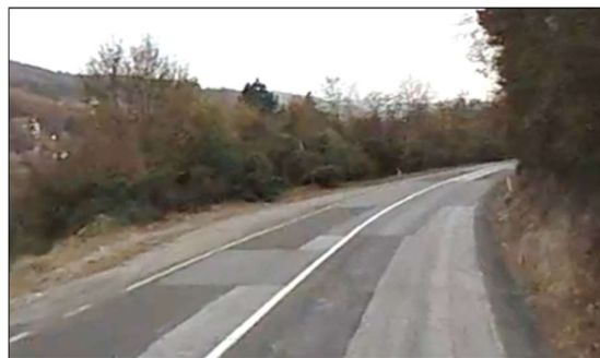
Picture 43. Damage of pavement
