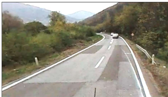
Picture 42. Damage of pavement
