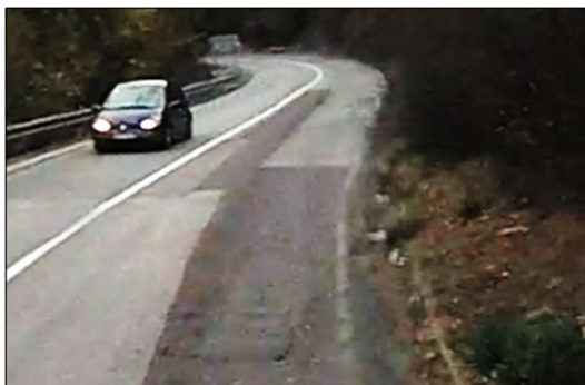
Picture 44. Damage of pavement
